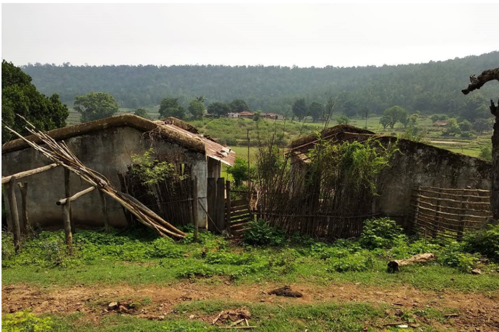
Poor quality of houses built under the Birsa Awas Yojana
