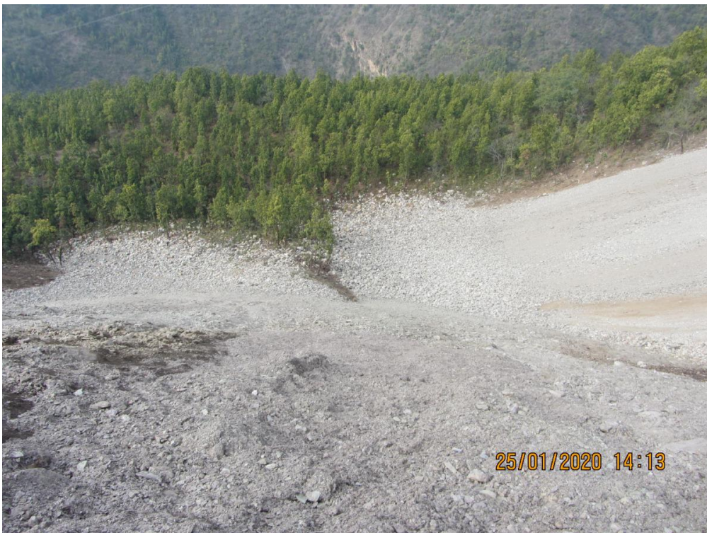
Debris from high cutting carelessly dumped by a forest on NH-125
