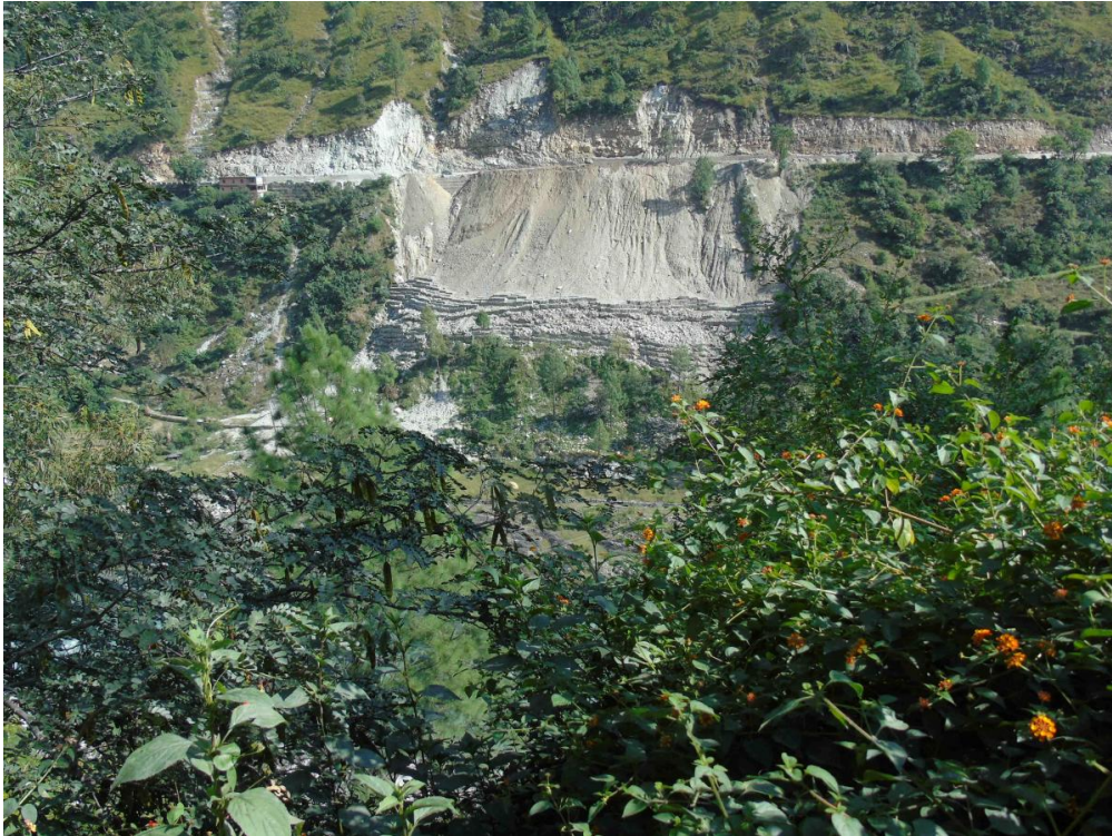
Collapsing retaining wall at a muck dump on the Badrinath highway (NH-58)
