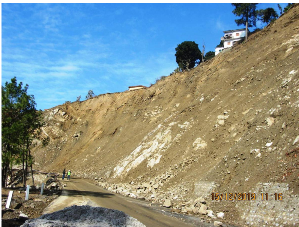
Debris overtop a token slope protection wall on NH-125
