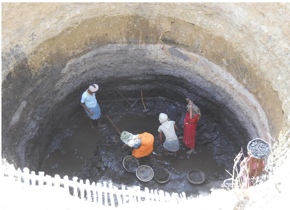
Well construction under the MGNREGS in Jharkhand: India's MGNREGS has been studied with RCTs | Photo: Manoj Dutt
